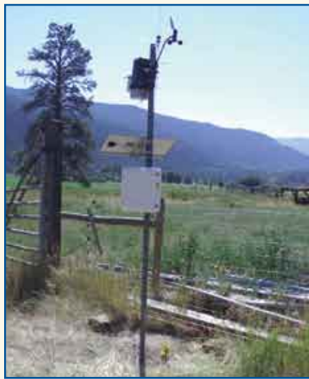
A Davis Vantage Pro2 Climate Station installed on Kane Lake Ranch near Merritt in the summer of 2005, to assist with water conservation efforts.
