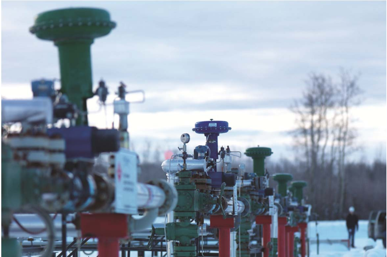
In BC's Northeast – Natural gas handling facility
