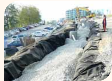
Photos: (Top) Green roof and (Bottom) infiltration trench construction and UniverCity Community Development, Burnaby, BC.
